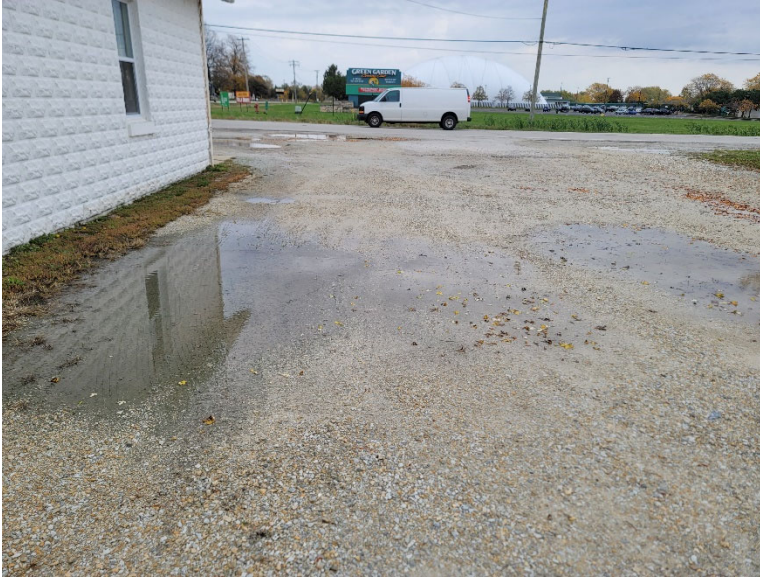
Figure 3 Ponding of water in parking lot
