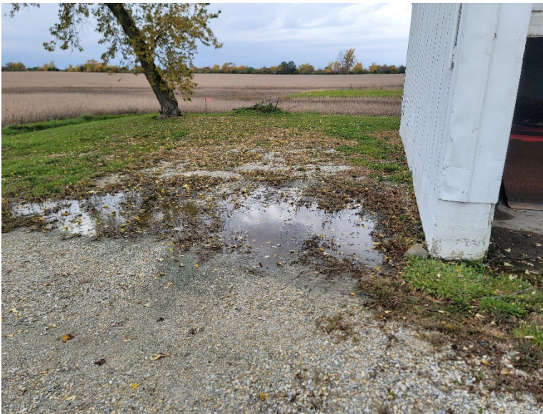
Figure 2 Ponding of water adjacent to Barn
